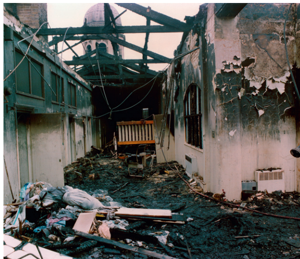
Figure 11 An example of a typical heat horizon. Photo courtesy of Mick Gardiner, Gardiner Associates, with permission. Copyright 2012 from Scientific Protocols for Fire Investigation , 2nd Edition by John J. Lentini. Reproduced by permission of Taylor and Francis Group, LLC, a division of Informa plc.
