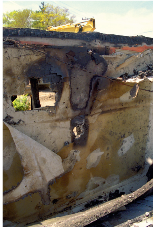
Figure 13 Opposite side of the wall shown in Figure 12 . The outline of the stud space can be clearly seen. Copyright 2012 from Scientific Protocols for Fire Investigation , 2nd Edition by John J. Lentini. Reproduced by permission of Taylor and Francis Group, LLC, a division of Informa plc.
