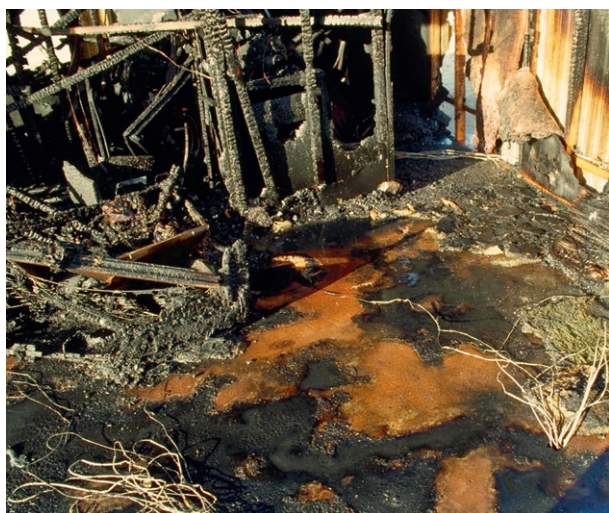
Figure 16 A more typical irregular pattern caused by the random failure of the carpet, resulting in alternate areas of exposed and protected subflooring. Copyright 2012 from Scientific Protocols for Fire Investigation, 2nd Edition by John J. Lentini. Reproduced by permission of Taylor and Francis Group, LLC, a division of Informa plc.
