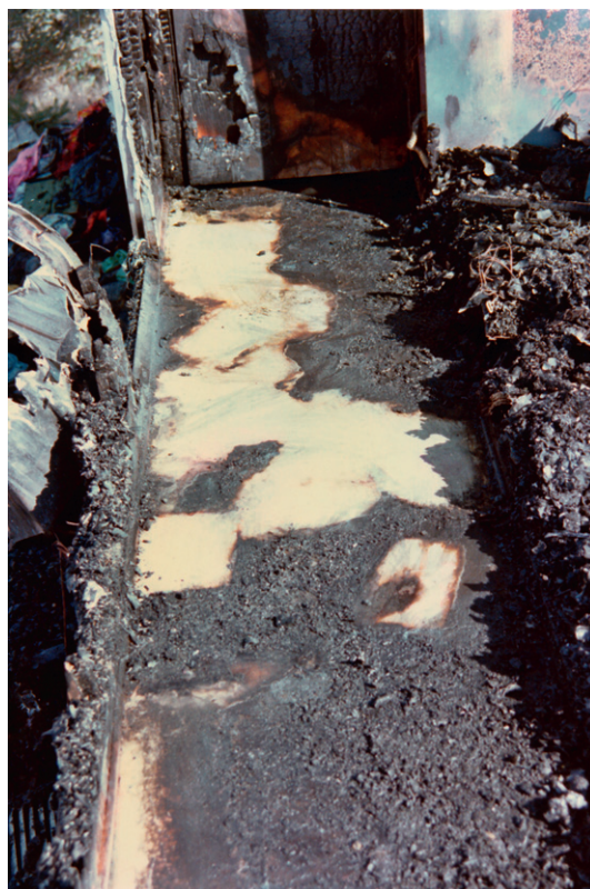
Figure 17 This fire pattern was erroneously attributed to the burning of ignitable liquids. The unburned areas were protected by objects on the floor. Photograph courtesy of David M. Smith, Associated Fire Consultants, with permission.
