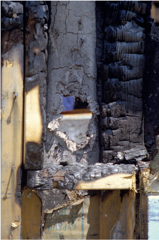
Figure 12 An example of a horizontal confinement pattern. Hot embers from above fell onto the horizontal member, where they caused damage to the drywall. Copyright 2012 from Scientific Protocols for Fire Investigation , 2nd Edition by John J. Lentini. Reproduced by permission of Taylor and Francis Group, LLC, a division of Informa plc.
