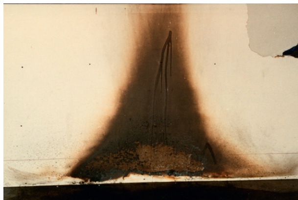
Figure 2 Triangle-shaped pattern, also called an inverted cone pattern, produced in a test fire. Copyright 2012 from Scientific Protocols for Fire Investigation , 2nd Edition by John J. Lentini. Reproduced by permission of Taylor and Francis Group, LLC, a division of Informa plc.
