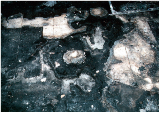
Figure 18 This fire pattern was erroneously attributed to the burning of ignitable liquids. The unburned areas were protected by objects on the floor.
