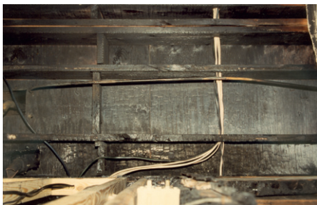
Figure 9 Semicircular pattern on the underside of the floor above the origin. The fire originated at an overheated switch inside the wall cavity. Copyright 2012 from Scientific Protocols for Fire Investigation , 2nd Edition by John J. Lentini. Reproduced by permission of Taylor and Francis Group, LLC, a division of Informa plc.
