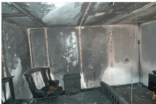
Figure 21 Clean burns resulting from a short-lived test fire. The wall between the bed and the chair never accumulated any soot. The wall and ceiling above the nightstand were damaged by the burning of a fuel-rich cloud of smoke produced by the chair. Photo courtesy of ATF Fire Research Laboratory and Steven W. Carman, Carman Fire Investigations, with permission.
