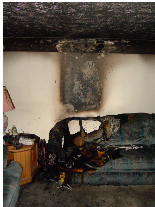
Figure 4 A columnar fire pattern produced by a fire that was extinguished prior to the formation of a V-shaped pattern. Copyright 2012 from Scientific Protocols for Fire Investigation , 2nd Edition by John J. Lentini. Reproduced by permission of Taylor and Francis Group, LLC, a division of Informa plc.
